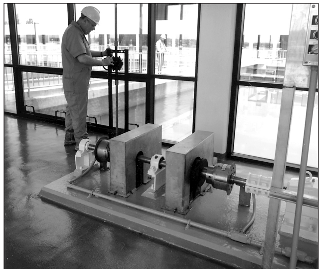
H1900 OVERLOAD CLUTCH WATER TREATMENT PLANT
