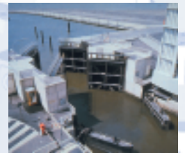
deva.metal ® , deva.glide ® in sluice construction: double lock: neck- and step bearings
