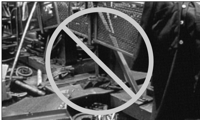
Don't clutter area around belt drive
