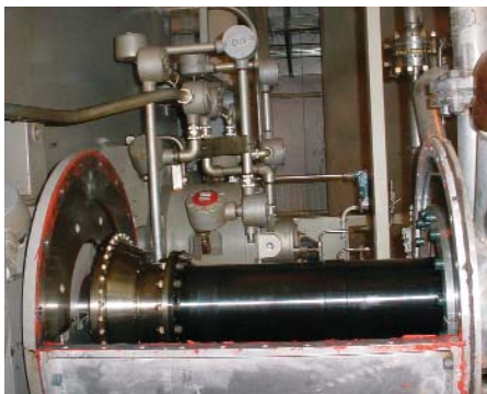
Figure 7: A coupling spacer blackened by "smoking" hot oil from nearby bearing housing. The oil got heated by an overheated coupling guard
