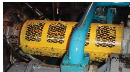
Figure 10: Expanded metal coupling guard protects personnel
