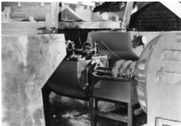
DBZ coupling on a soot blower in a power plant.
