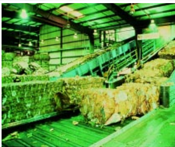
Paper bale handling conveyor system.
