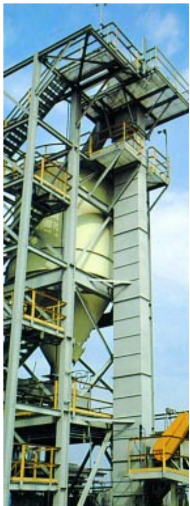
Bucket elevator installation at a fertilizer plant.
