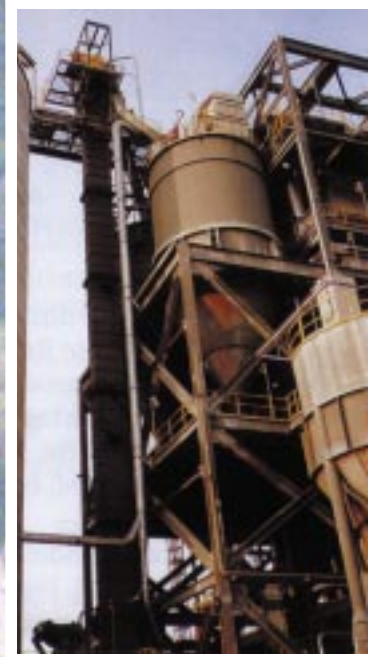
Bucket elevators at a coal-fueled power plant.
